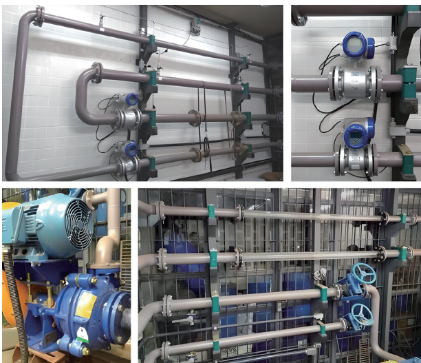
Fig. 1 Test-loop experimental facility.
